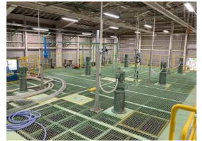
Upgraded pit wastewater treatment facility (Komagi Mine)
